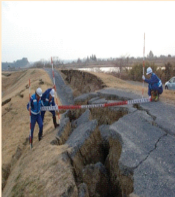
FIGURE 2: Damage to the river dikes at Narusegawa
